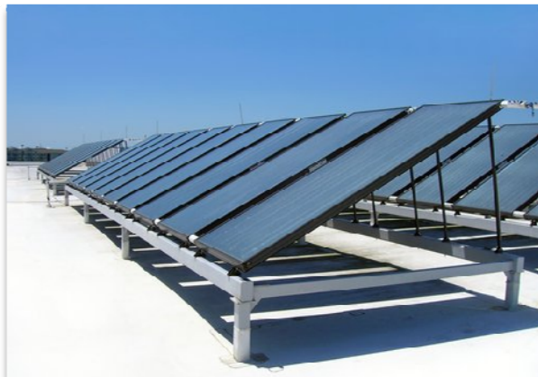
Large Scale Solar Thermal Installation 1
