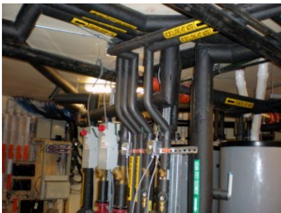
Interior Solar Hot Water Piping 2
