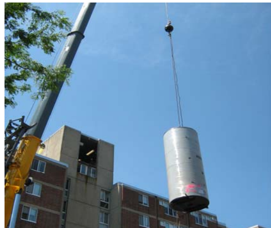
Solar Storage Tank at Castle Square Apartments, Boston, MA 3
