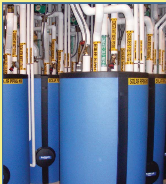
Fifteen Buderus hot-water storage tanks, with a maze of piping, were installed in a very confined pre-existing space in the RCF Boiler Room.
