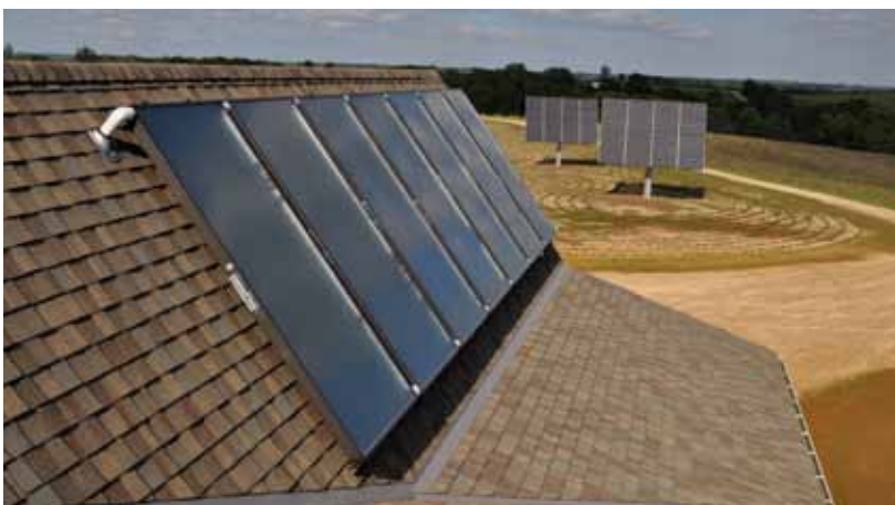
Residential solar hot water with ground-mounted PV in Viola, Wisconsin
