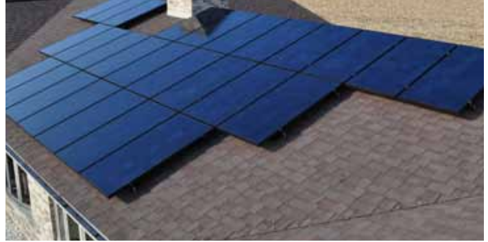
Residential solar installation in Columbus, Wisconsin
