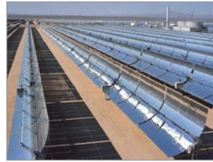
Parabolic trough technology
