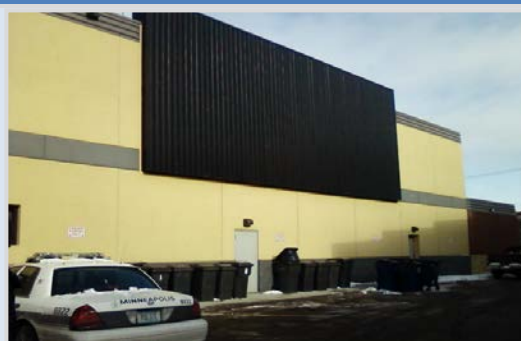
Figure 5. Solar wall on the south side of the 3 rd precinct police station.
