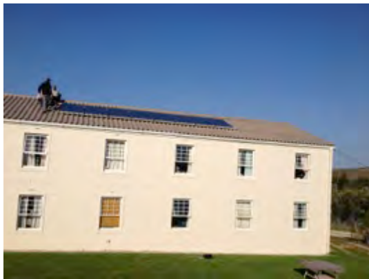
Figure 7: Typical multi family building solar water heater installation
