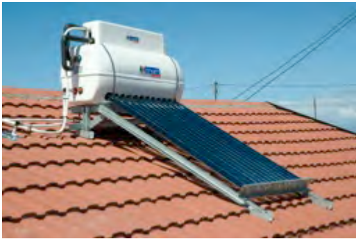
Figure 5: Typical gravity fed / low-pressure solar water heater with evacuated tube collector
