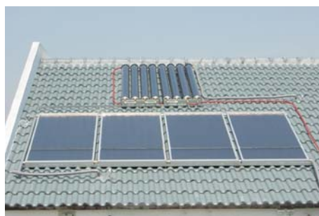
(a) Integration of solar collectors with cement tile roofing
