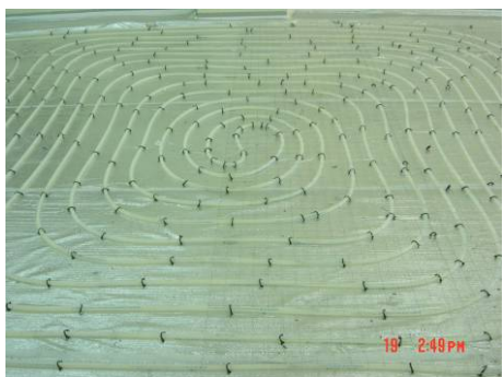
Fig. 21 Photo of floor heating coil pipes
