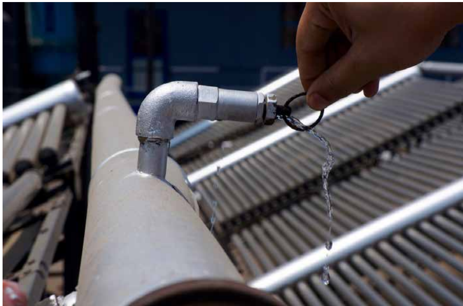
Figure 3 Vent valve to remove air from the collector circuit
