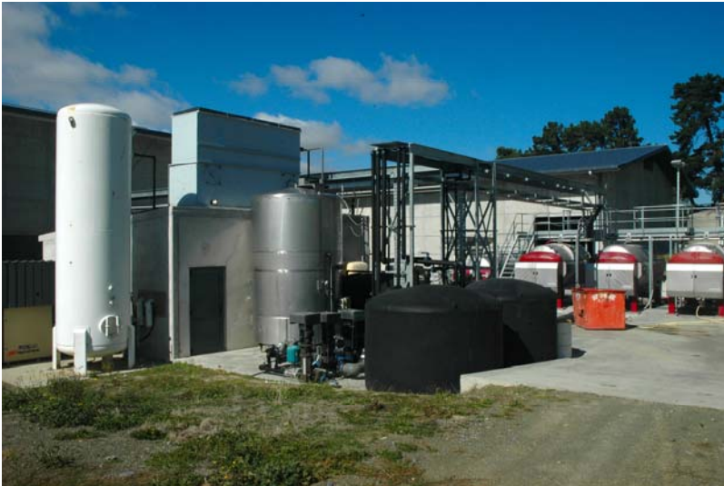
Photo 1. Storage tanks for cold (stainless steel) and warm glycol (plastic).
