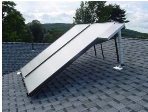
Roof top solar collectors on the Massachusetts home.
