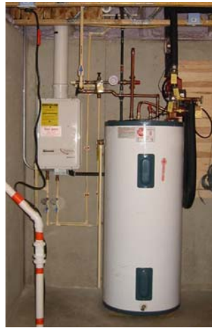
Auxiliary tankless gas water heater and solar storage tank in basement of Wisconsin home.
