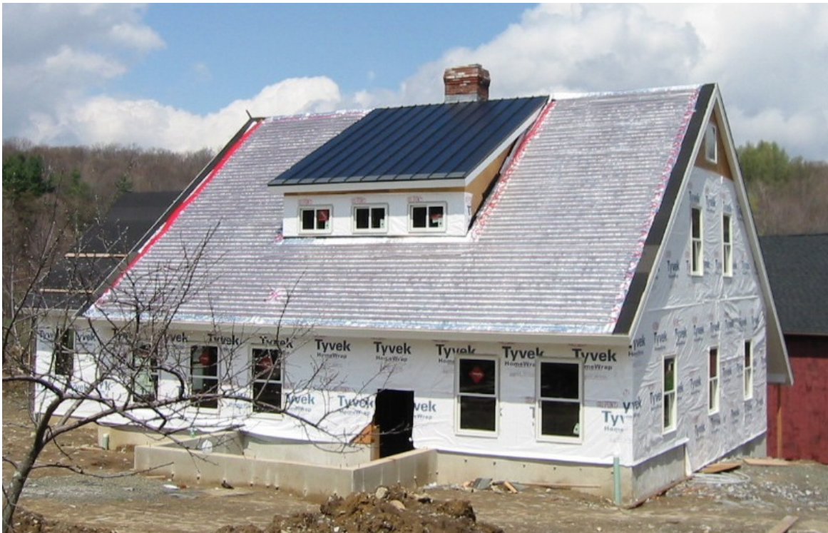
Fig. 2: The solar thermal collection system installed on main section of southern roof consists of red PEX tubing and metal heat transfer channels. On the shed dormer, the standing-seam metal roof and PV laminates have already been installed over the thermal collection components.
