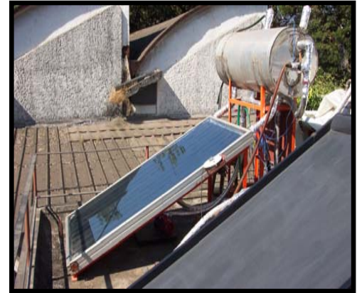
Test Facility for thermosyphon systems
