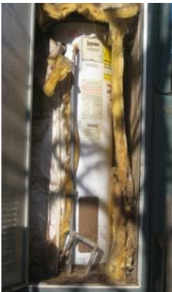
Figure 4: Electric water heater in the PPN
