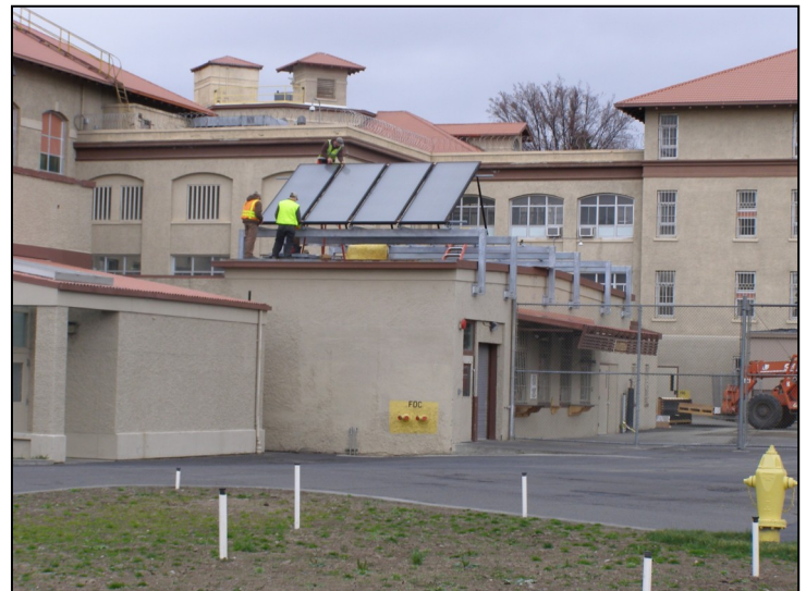
A solar thermal system is more reliable and requires less maintenance than a domestic hot water system for Eastern Oregon Correctional Institution in Pendleton. It was paid for in part with Recovery Act (stimulus) funding from the Oregon Department of Energy.
